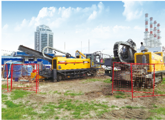
XZ680A working for the gas pipeline construction in Russia, weathered rock stratum
